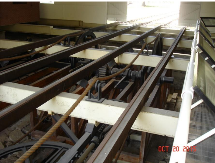
Gearing and sheaves on the inside of the rebuilt and restored engine house at the top of Incline #6. Note the rope and the flat iron bars on top of the wooden rails.
