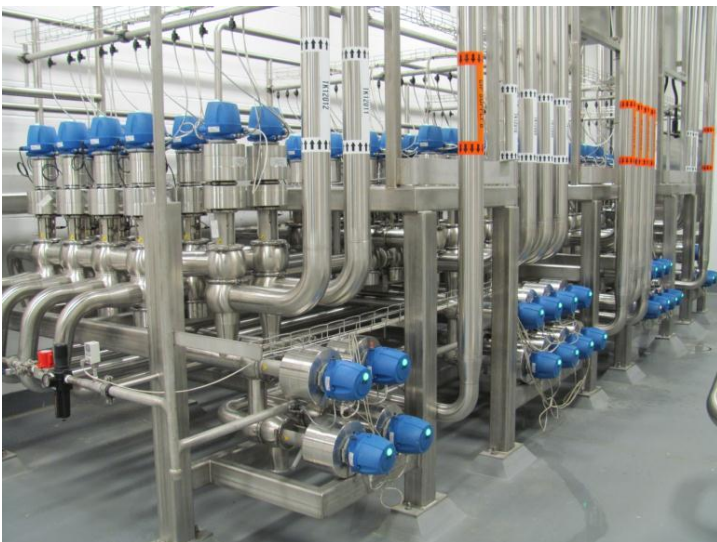
Sample of the more than seven miles of stainless steel piping and 1,609 control valves
