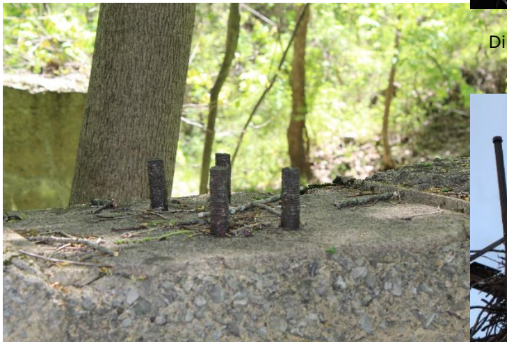
Top of piers. Note condition of concrete after over 100 years.
