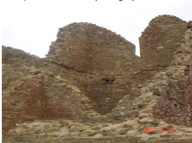
A rather formidable structure! Note the wooden beams that supported a second story.
