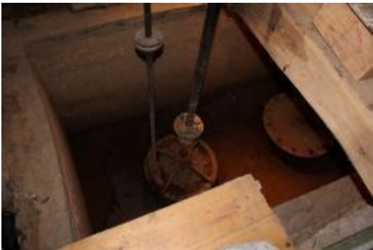
The two turbines, in the basement of the building. Water flowed horizontal.
