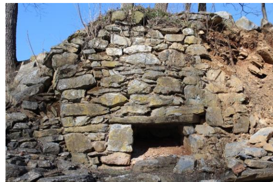
Also on River Road. This could be an old lime kiln, or maybe a pizza oven?
