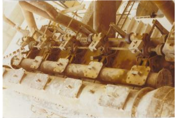
Mechanical monstrosity dust collector bag shakers.
